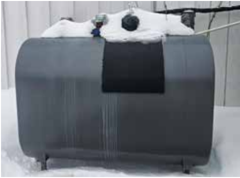
Figure 3 Outside steel tank at Entech with added top insulation pad by fuel line pass-throughs
