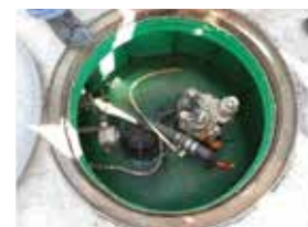
Sump pump as shown by Fuels Market News
